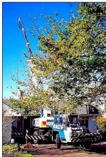
The crane lifting trees from the rear yard to the front of the house
